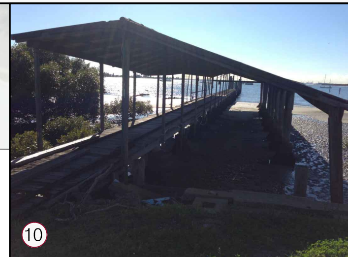
10 HERITAGE JETTY. BIRD ROOSTING ON THE ASBESTOS ROOFING. NEEDS REFURBISHMENT AND SCREENING.
